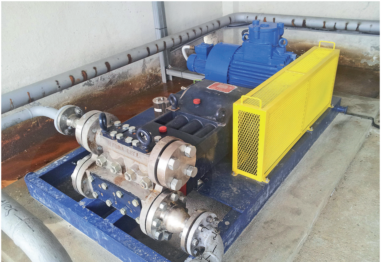
Hydra-Cell T8045 pump installation at a plant of OMV Petrom in Romania
